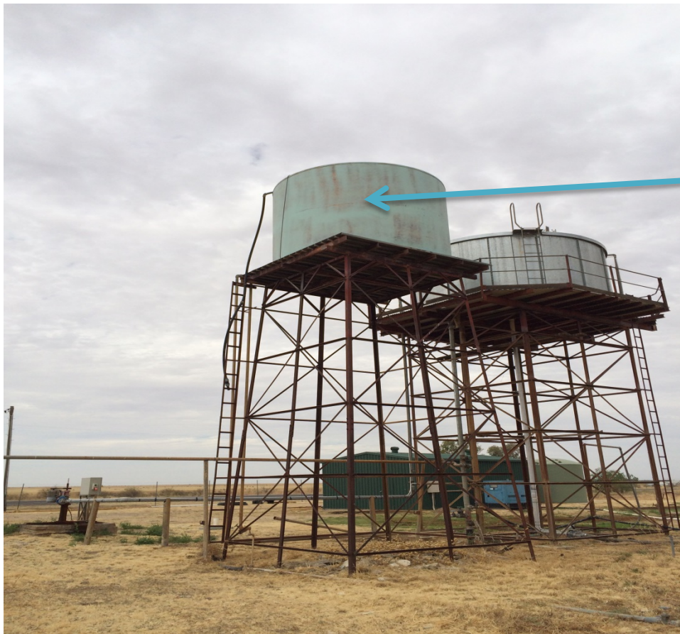
Fibre glass tank on steel truss or similar stand, to be dismantled and disposed of – even though this tank is no longer in use there is still interconnecting pipe works that will need to be blinded off/removed before the structure is demolished – this will need to be undertaken in consultation with Council Plumbers – North eastern view
