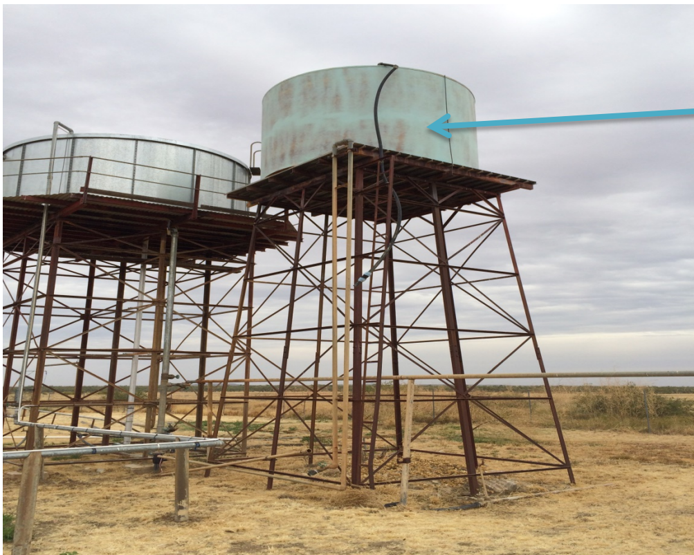
Fibre glass tank on steel truss or similar stand, to be dismantled and disposed of – South eastern view
