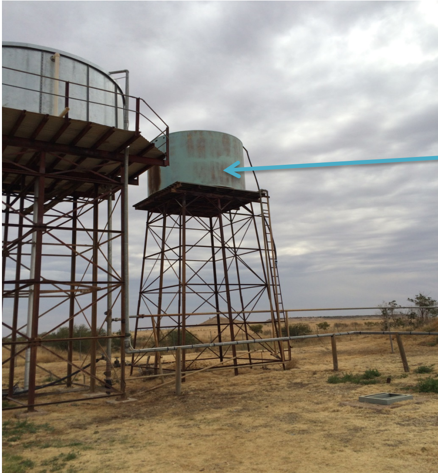
Fibre glass tank on steel truss or similar stand, to be dismantled and disposed of – South western view
