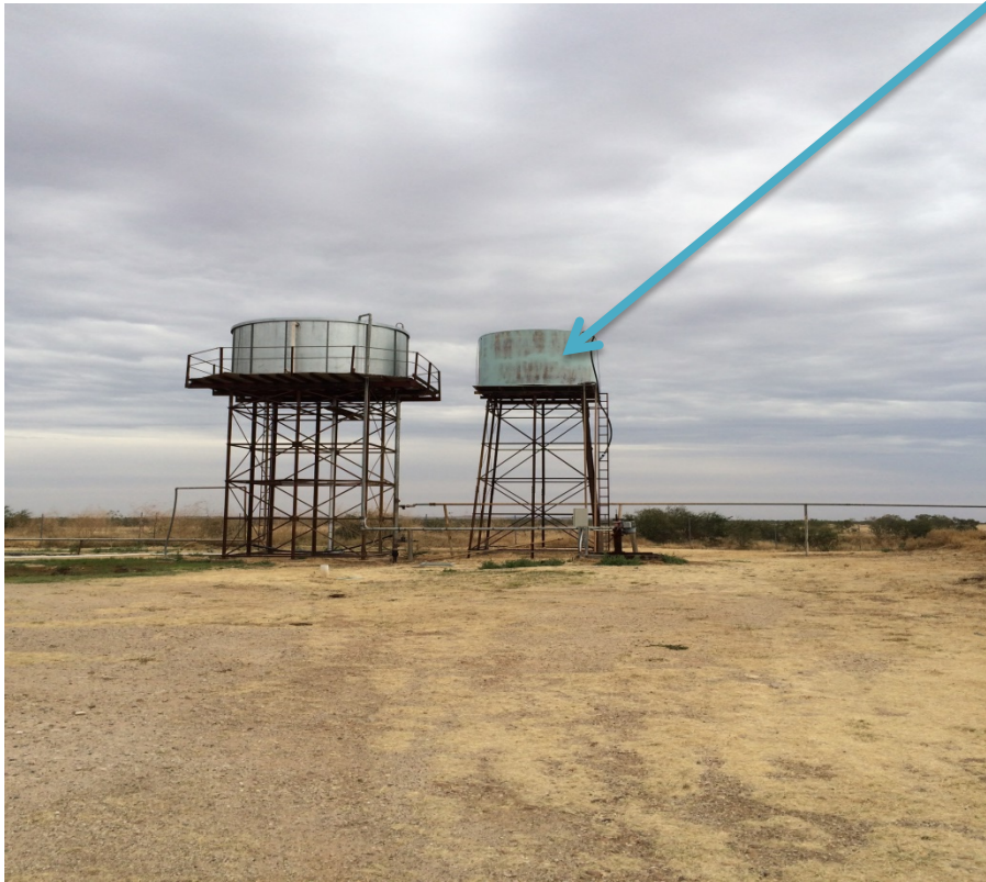
Fibre glass tank on steel truss or similar stand, approximate height 8m from base of tank to ground level – This tank and stand is to be dismantled, removed and disposed of – the tank is abandoned and no longer in service – Southern view
